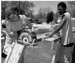
In YouthBuild programs, low-income young people ages 16 to 24 work full-time for 6 to 24 months toward their GEDs or high school diplomas while learning job skills by building affordable housing in their communities. Photo
